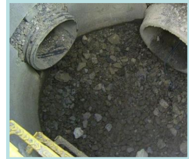
M3 Clonee to Kells: Manhole.
