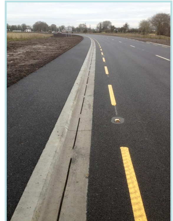
Nearside linear drainage channels.
